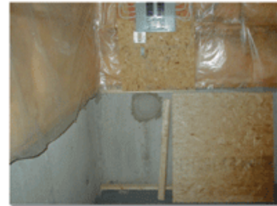
Notice the patched hole in the foundation below the electrical panel where stolen power was brought into the home.
